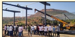
Joshi construction plant, Satara.
